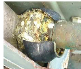
Galvanic corrosion under the plastic sleeve.
