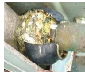
Galvanic corrosion under the plastic sleeve.
